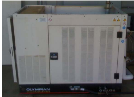
Figure 3.1 Generator Outside View
