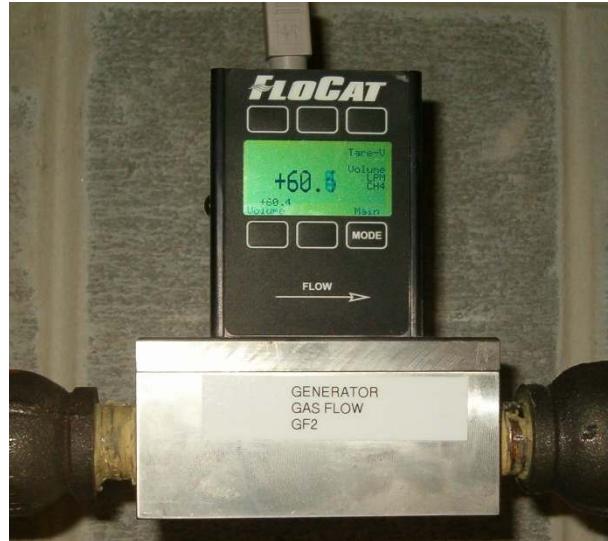
Figure 3.15 Natural Gas Flowmeter
