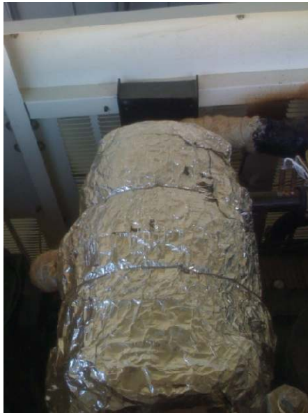
Figure 3.3 Exhaust-Coolant Heat Exchanger
