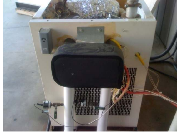
Figure 3.4 Coolant-Heat Recovery Heat Exchanger
