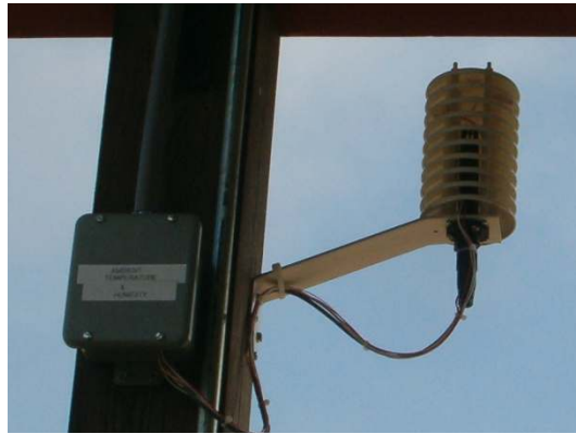
Figure 3.18 Ambient Relative Humidity Sensor
